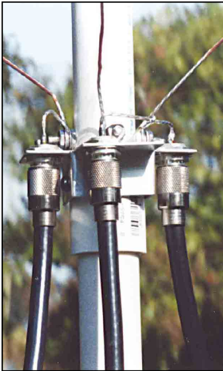
A close-up view of the base and connector assemblies. The photo preceded the final waterproofing of all exposed connections.
